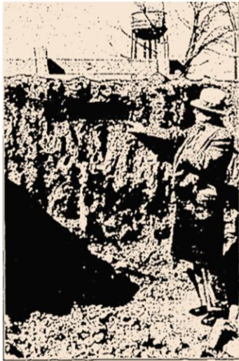
EXCAVATIONS for the new nurses' home at the county hospital have revealed that it is being built on an abandoned potter's field. Vincent Pacholski, one of the contractors, is shown beside a hole which formerly held a small baby's coffin.—Journal Photo
